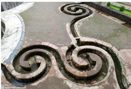
Fig. 4. The spiral channels that would slow down and filter the water before it entered the Kund [6]
